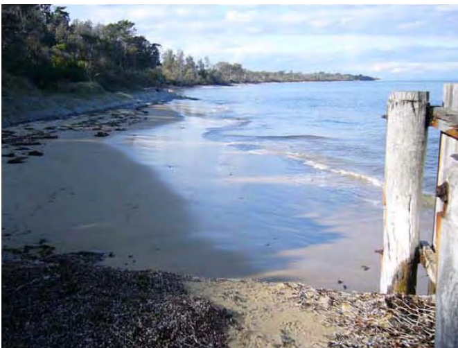
Erosion beyond eastern end of sea wall
